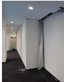
Before repair (6F apart)
