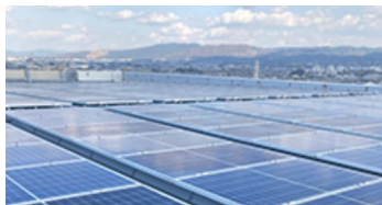
Tenri Distribution Center (Power generation capacity: 100.00kW)
