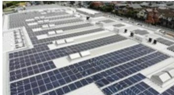
Kawamachi Yahagi Mall (Power generation capacity: 302.40kW)
