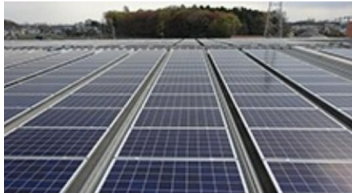
Unicus Ina (Power generation capacity: 334.53kW)
